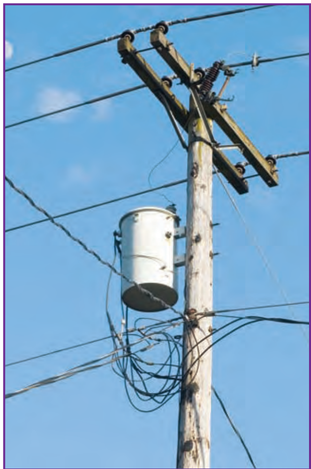
Devices called transformers use magnetism to lower the voltage to the 120 V used in homes.
