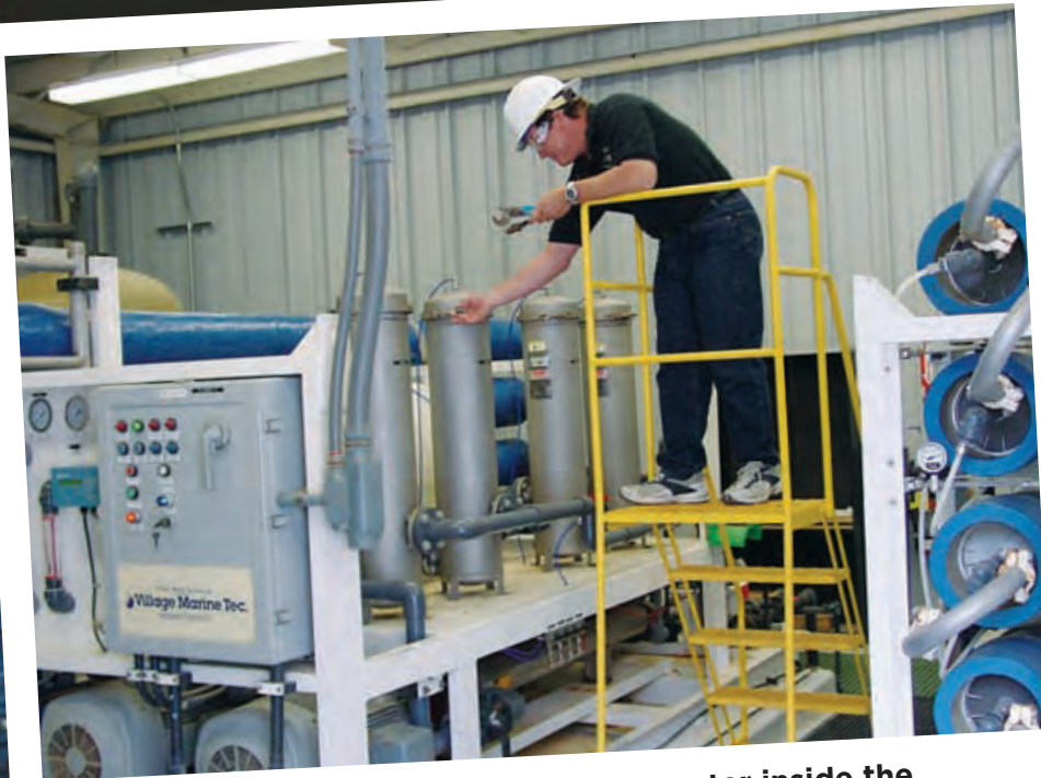
Salts are removed from ocean water inside the Santa Catalina Island desalination plant.
